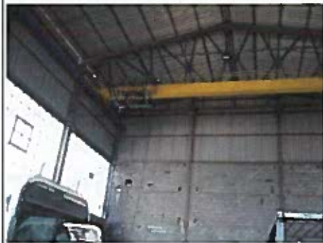
Workshop Bulk and General Cargo – Overhead crane main hall
